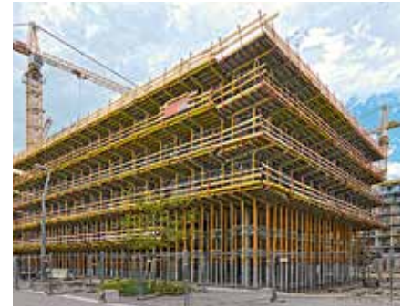
The PERI solution with MULTIPROP and MULTIFLEX, as well as for forming the circumferential balconies, served simultaneously as working scaffold.
