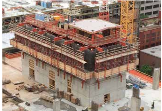
Integrated roofing for the climbing formwork accelerated the installation of the elevators by almost one year.
